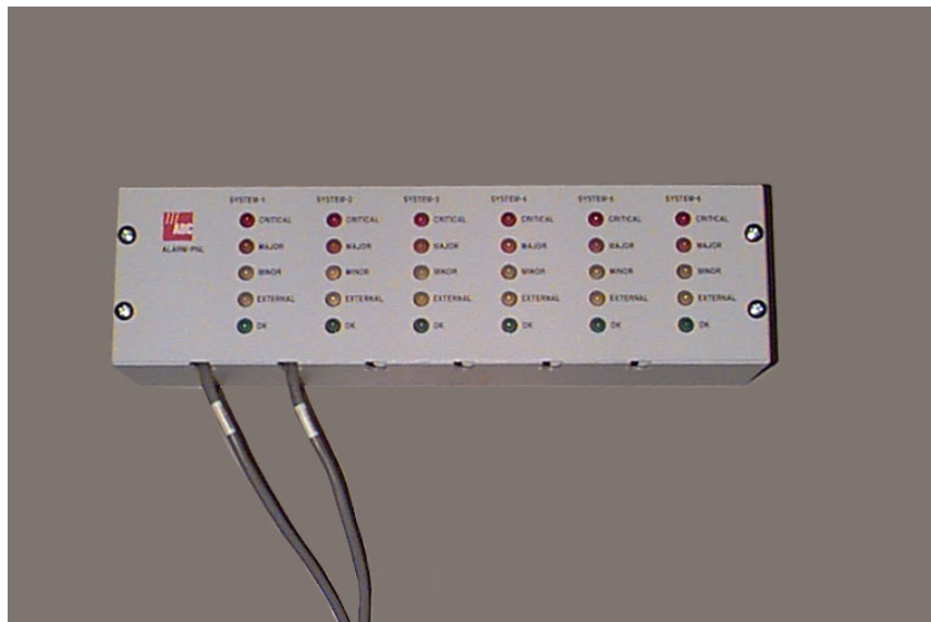
Figure 1. ALARM-PNL Panel Installed on the Wall
